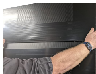
5. Position newly completed Mod Wall section on top of existing Wall structure
